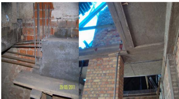
Figure 3: lightly frosted glass concrete
